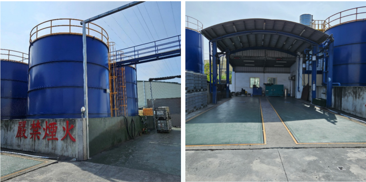
Audit of facilities handling waste oil-water mixtures
